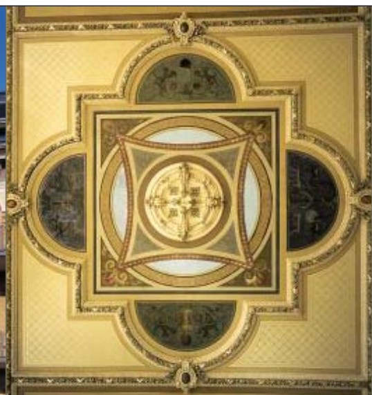
A close-up view of the lovingly restored ceiling in the former industrialist's villa
